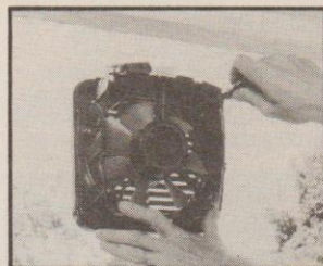
Screwing the Xpelair fan in the pane – you are cutting out some of the light but it's easier than installing a wall-mounted one
