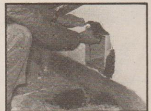
4: Cementing in the fan casing. Once the cement and surface plaster has dried and been redecorated, you should have a really neat finish
