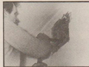
2: Chopping out bricks from the inside with a cold chisel and heavy hammer
