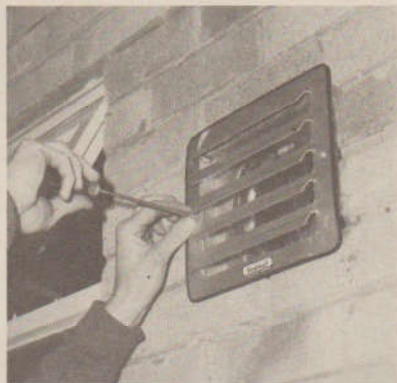
22. Outside louvre casing, in aluminium, is secured by screwing to the brickwork
