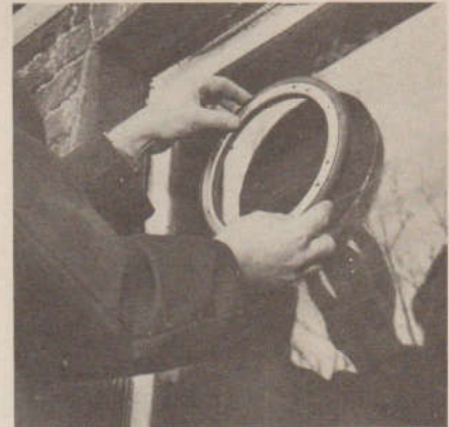
13. After circular hole is cut in pane the Thermor rim gasket is next fitted
