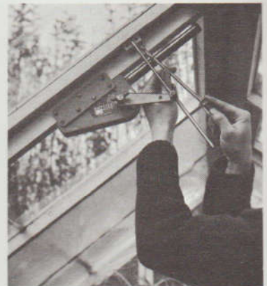
Fitting an automatic control—the Bayliss Autovent—to a ventilator. It can be adjusted to operate at a wide range of temperatures. There are special fittings for fastening the device to metal houses.
