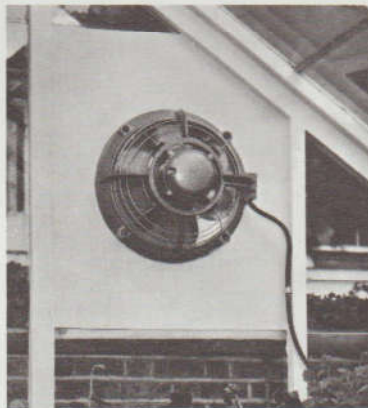
This extractor fan is mounted in a panel of resin-bonded plywood cut to match the pane that it replaces. To prevent chilling draughts, hinged louvres on the outside remain closed when the fan is idle.
